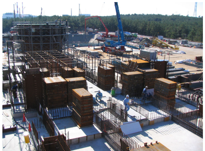
Status of the building construction for Muon Science Laboratory at J-PARC (December 1, 2004). The picture is looking from up-stream towards the neutron target station, in the foreground, several piles of 'built-in' iron blocks can be seen at the location of the MSL.
